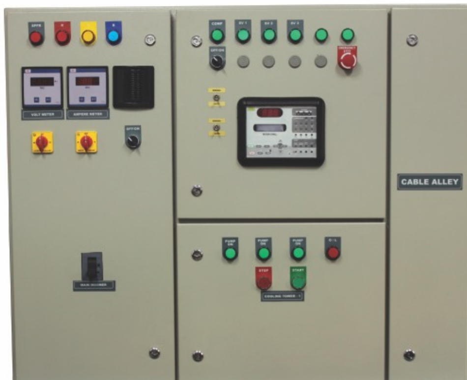
Process Chiller Electrical Panel
