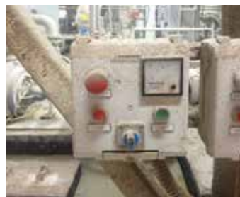
Enclosure used as a control unit in a fertilizer factory.
